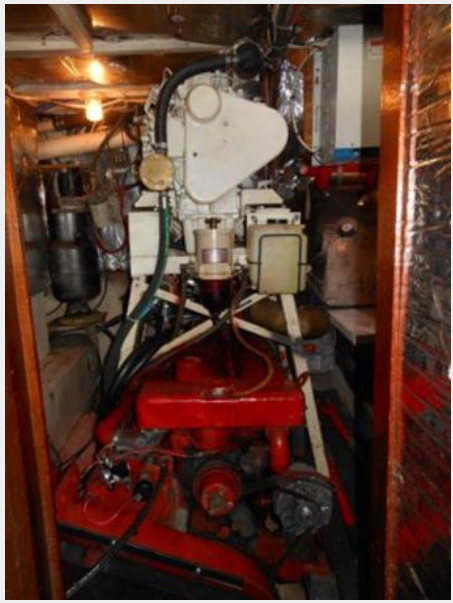
Generator above main engine
