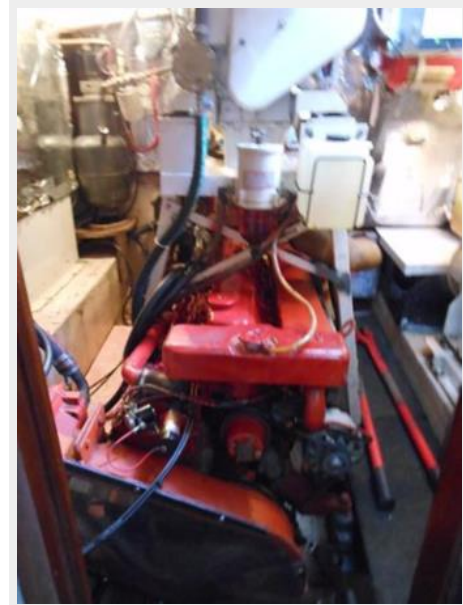
Main engine - 8KW generator above
