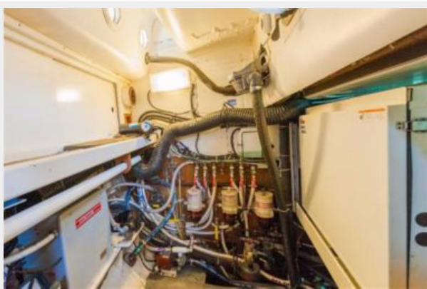
Standup Engine room - well planned
