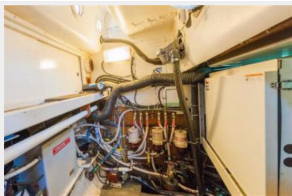
Standup Engine room - well planned
