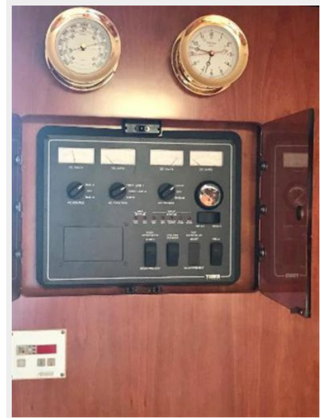
Shore Power/ Genset Panel
