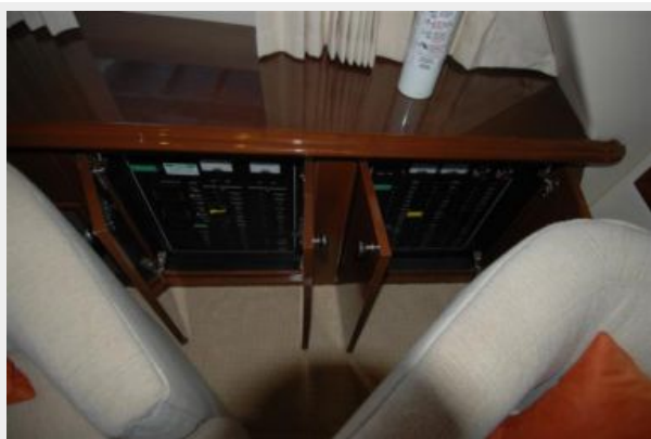
Salon Electrical Panel
