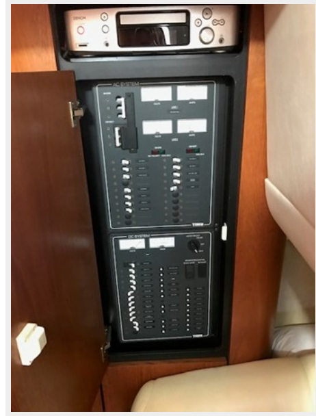
Main Distribution Panel
