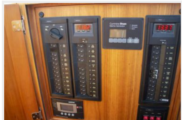
Main Electrical Panel
