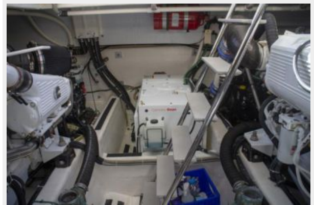
Engine Room Looking Aft
