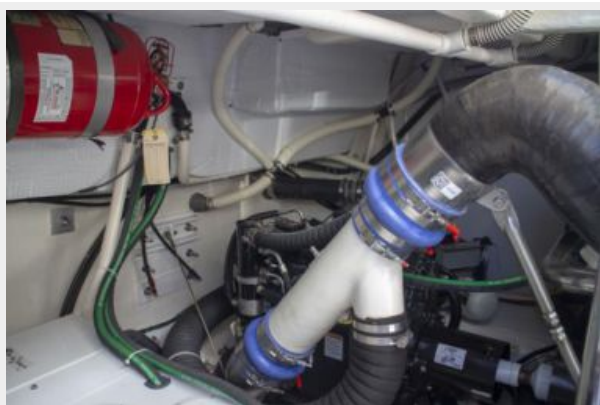
Fire Suppression System
