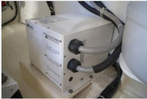
Shore Power Transformer
