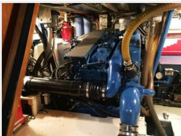
Very Clean Engine Room
