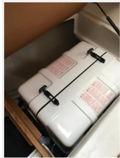
2004 Catalina 470 - Fischer panda generator
