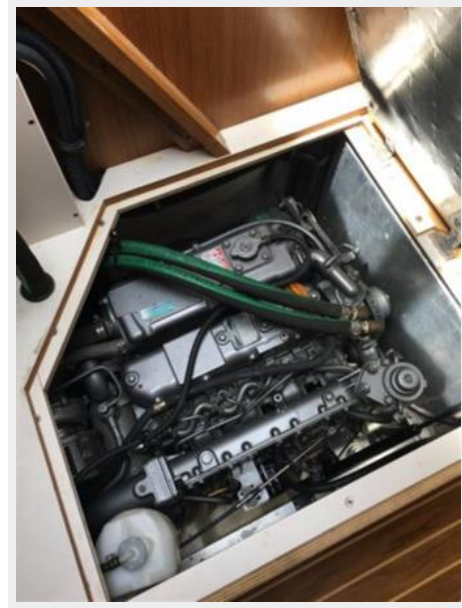
2004 Catalina 470 - Clean engine space
