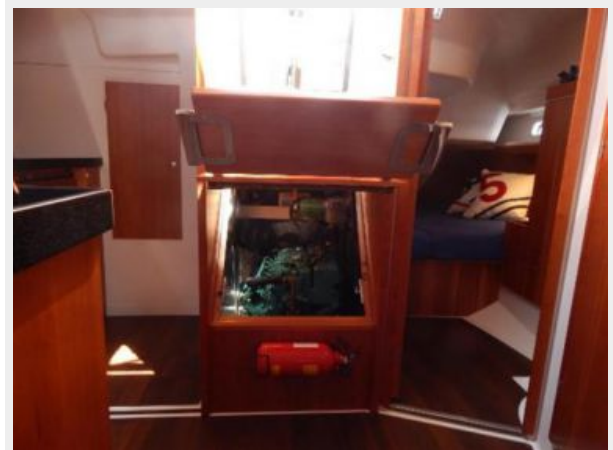
Engine room - under stairs
