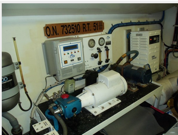
Outboard Starboard Engine
