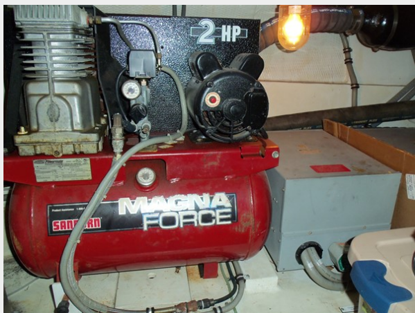
Starboard Side Gen Room
