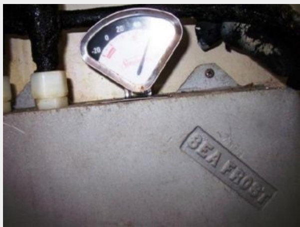
Galley_SeaFrost Refrigeration Cold-Plates
