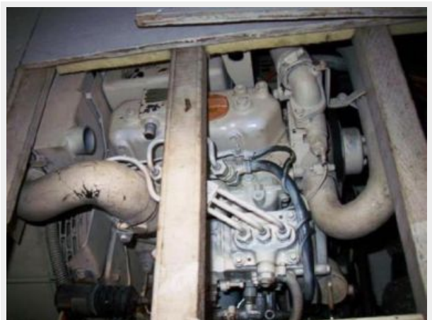
Kohler 5kW Generator Under V-Berth
