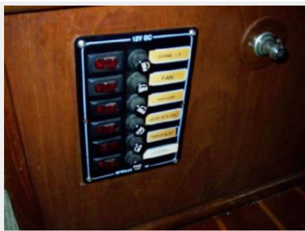
Electrical 12V Breakers
