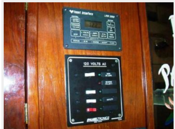
Link 2000 12V Controller & AC Additional Breakers
