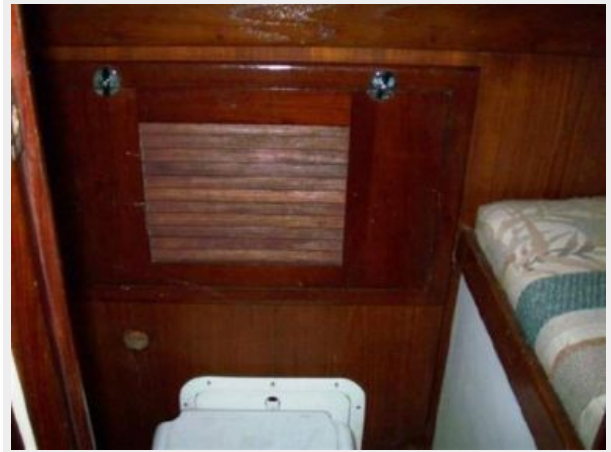
V-Berth_Generator Access Under Berth
