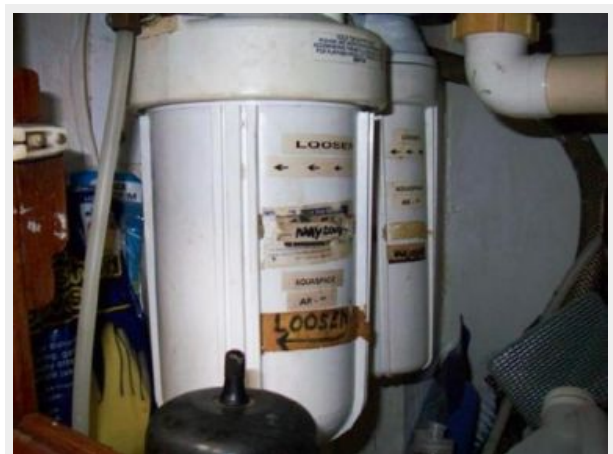
Water Filters under Galley Sink
