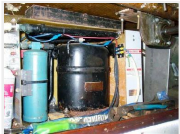
SeaFrost Refrigeration System
