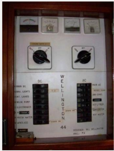
AC-DC Electrical Panel
