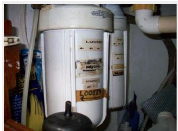
Water Filters under Galley Sink
