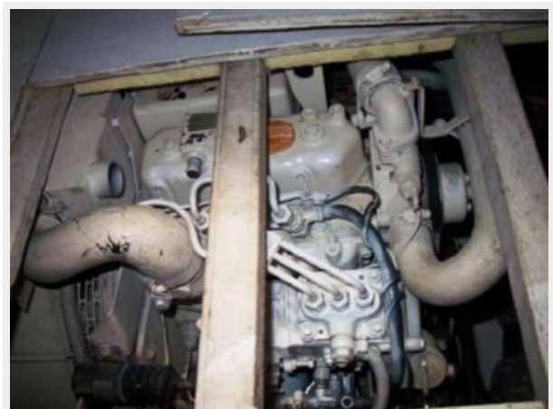
Kohler 5kW Generator Under V-Berth
