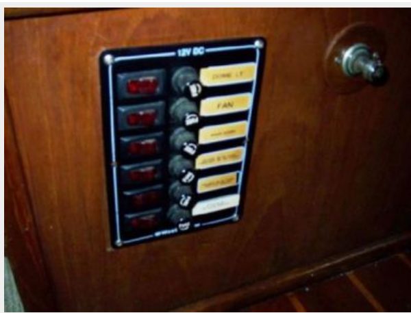
Electrical 12V Breakers
