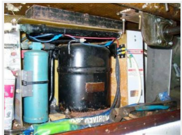
SeaFrost Refrigeration System
