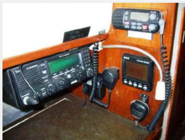
Nav Station Electronics
