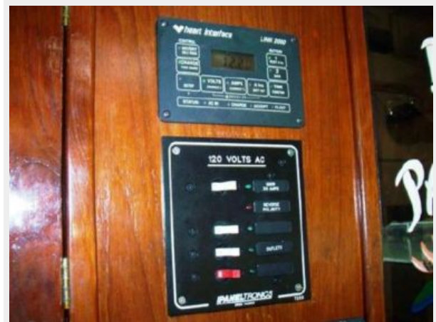
Link 2000 12V Controller & AC Additional Breakers
