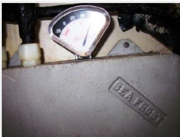
Galley_SeaFrost Refrigeration Cold-Plates
