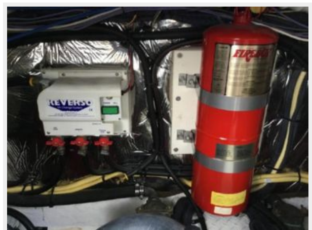
Oil Changer & Fire Suppression
