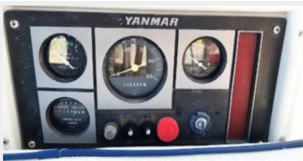
Main Engine Panel 5-4-18
