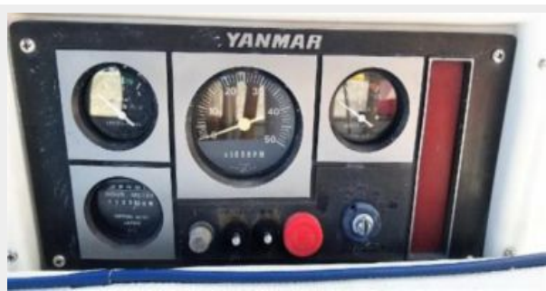
Main Engine Panel 5-4-18
