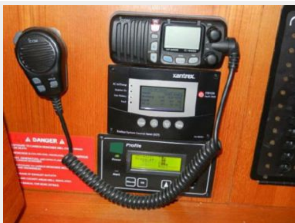
VHF, Xantrex monitor and Tank monitor
