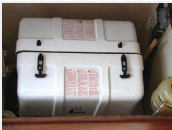
Fisher Panda Generator
