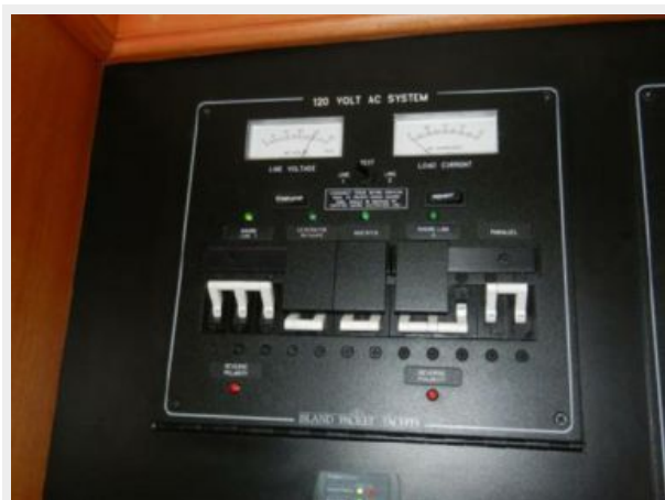
AC and Generator panel
