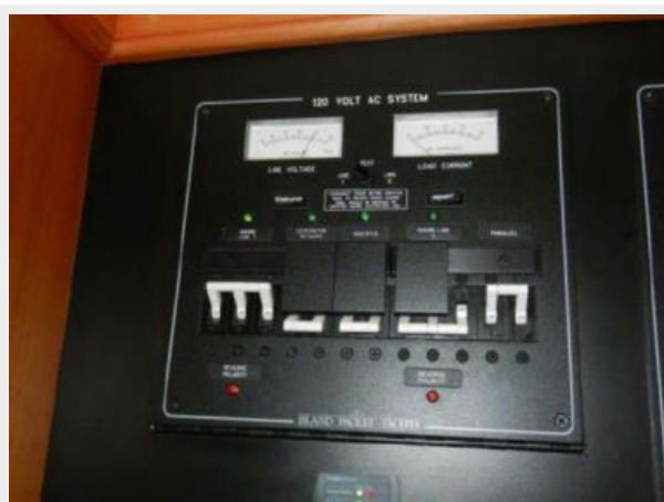
AC and Generator panel
