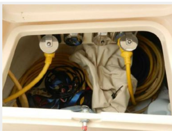
Shorepower plugs in locker
