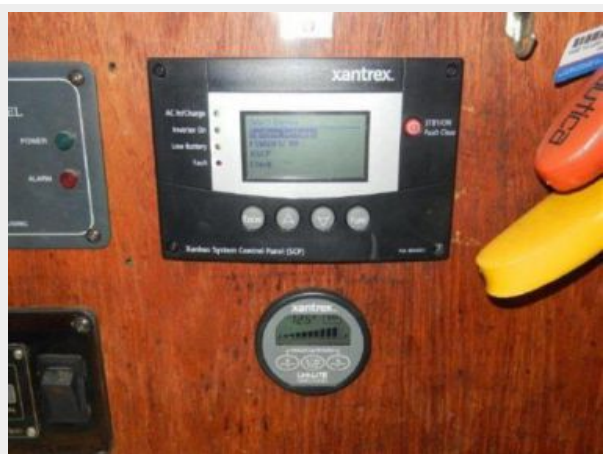
Xantrex panel for inverter and battery monitor
