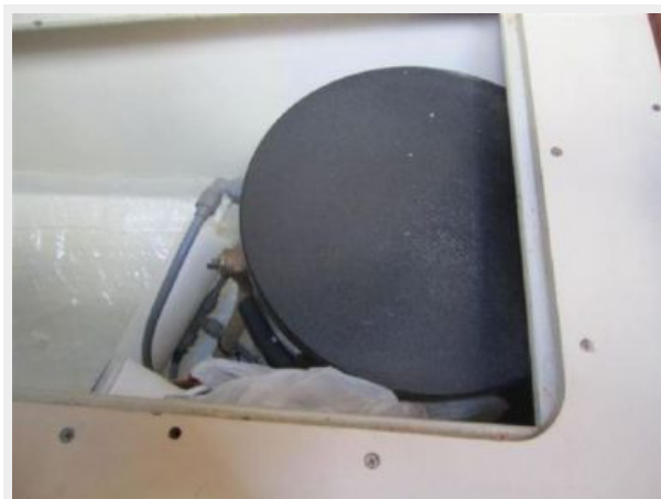
NEW WATER HEATER
