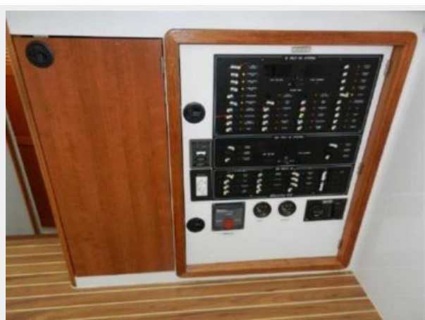
Electrical panel below chart table
