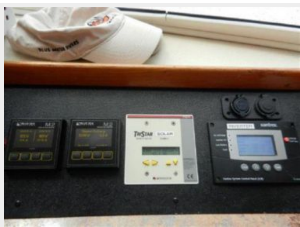
Solar control and battery monitors
