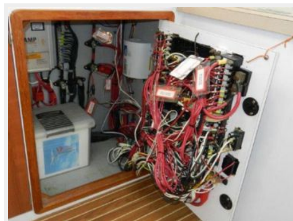
Wiring behind panel
