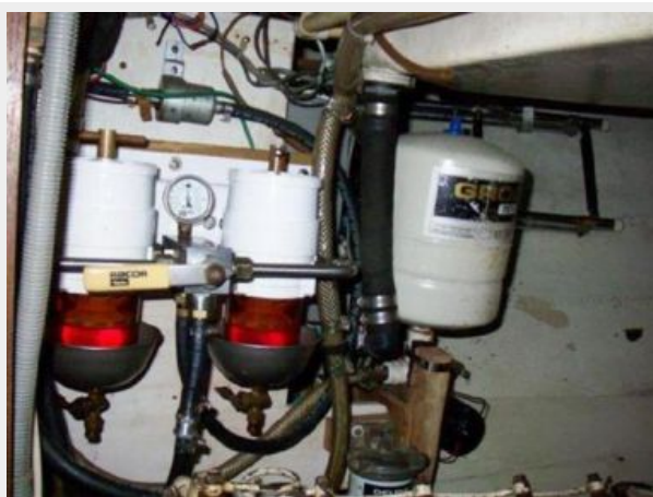
Engine room_Dual Racor Filters
