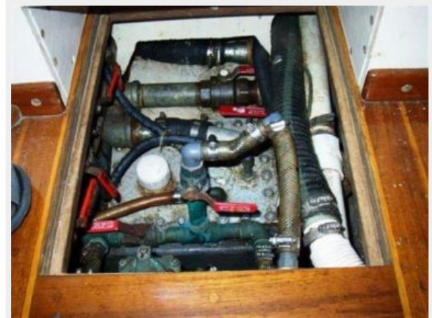
Fuel Tank Manifolds
