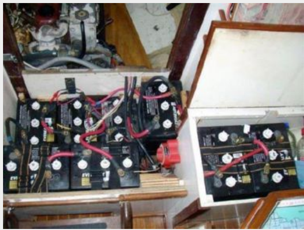
Batteries_Total of 740 Amp Hrs
