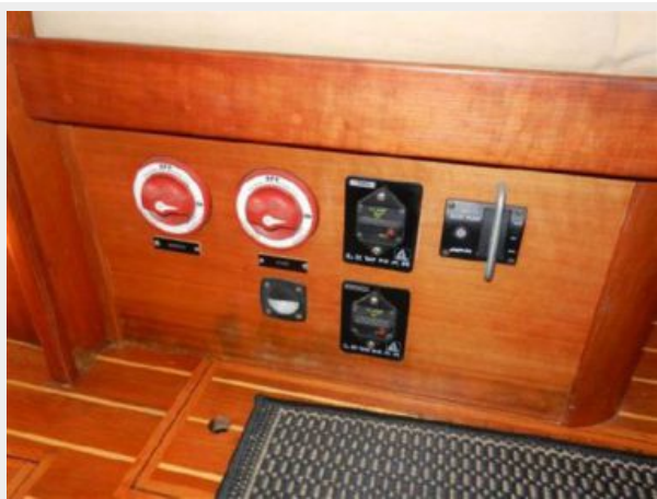
Battery switches and breakers
