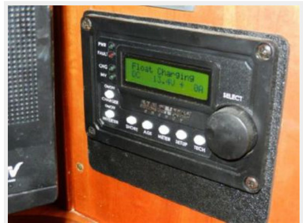
Magnum Energy battery monitor
