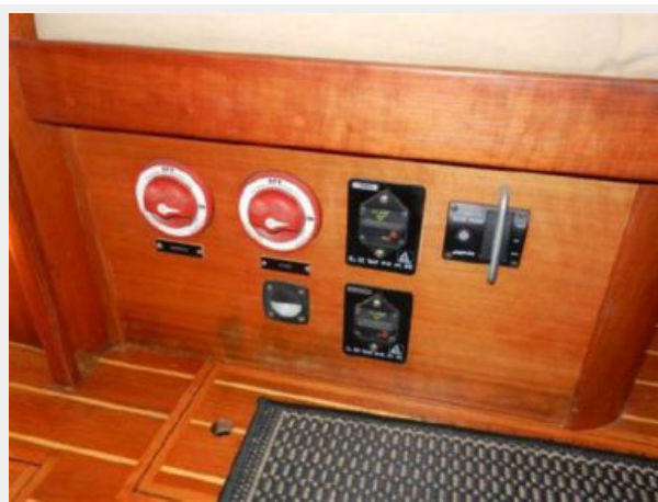
Battery switches and breakers
