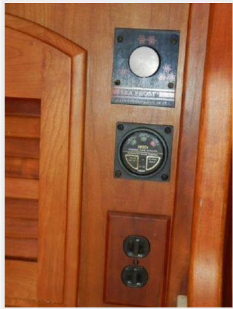
SeaFrost control, propane detector
