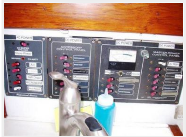
AC & DC Electrical Panels at Galley
