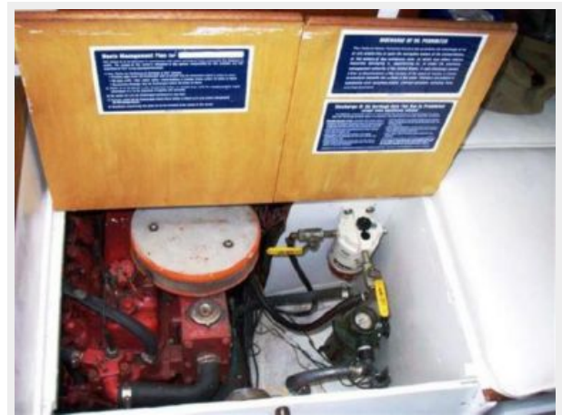
Engine Top Access
