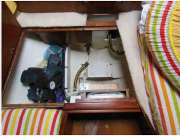
Forward Cabin anchor wash-down pump
