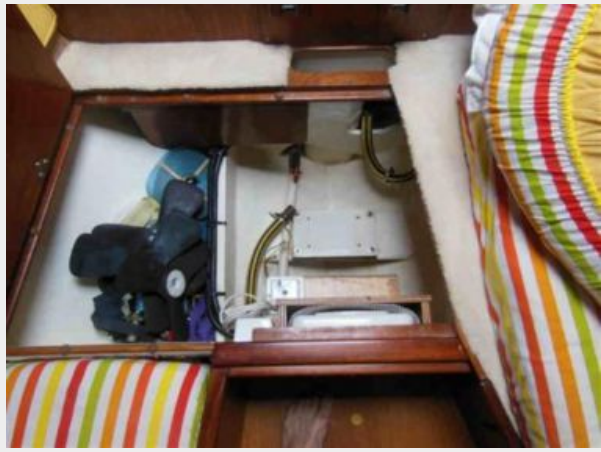
Forward Cabin anchor wash-down pump
