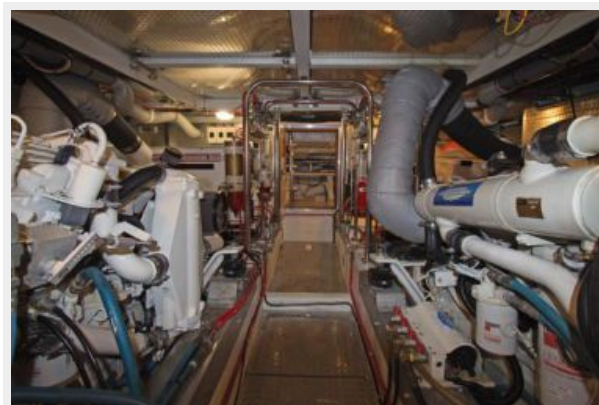
Engine Room Aft
