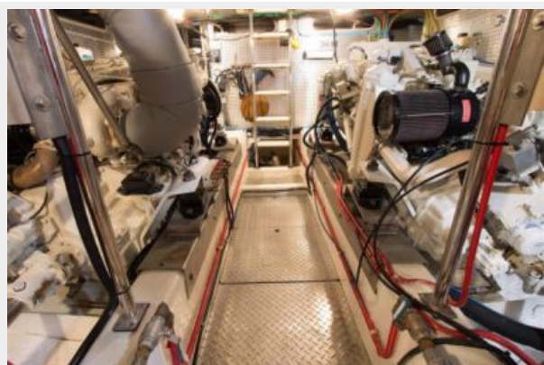
Engine Room Forward
