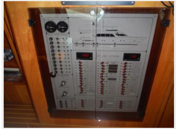
Pilothouse DC panel
