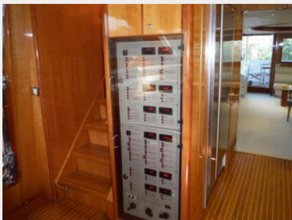
Pilothouse AC Panel
