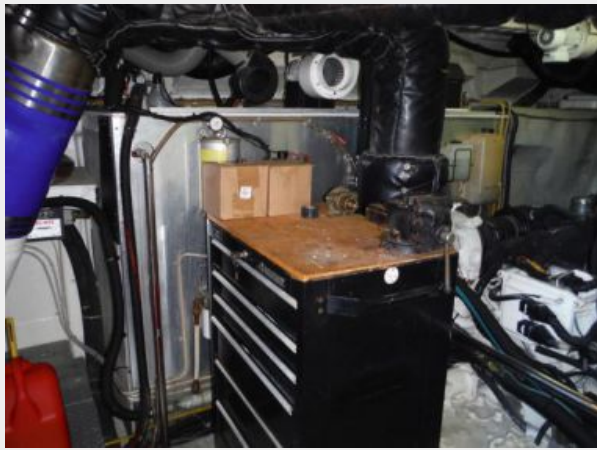
Aft of Port Engine
