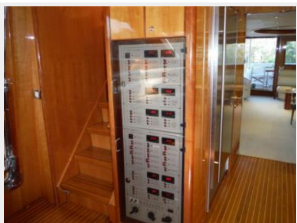
Pilothouse AC Panel
