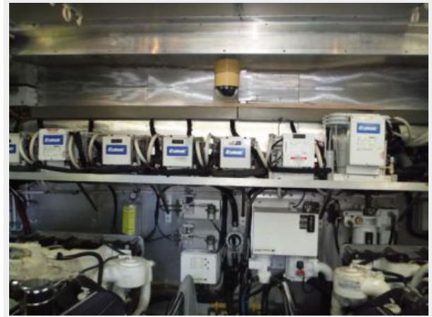
Engine Room Forward
