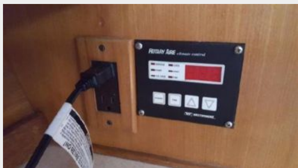
Air Conditioning Controls
