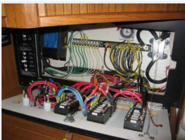
Clean wiring at electrical panel
