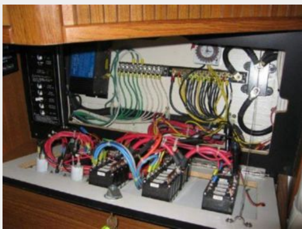
Clean wiring at electrical panel
