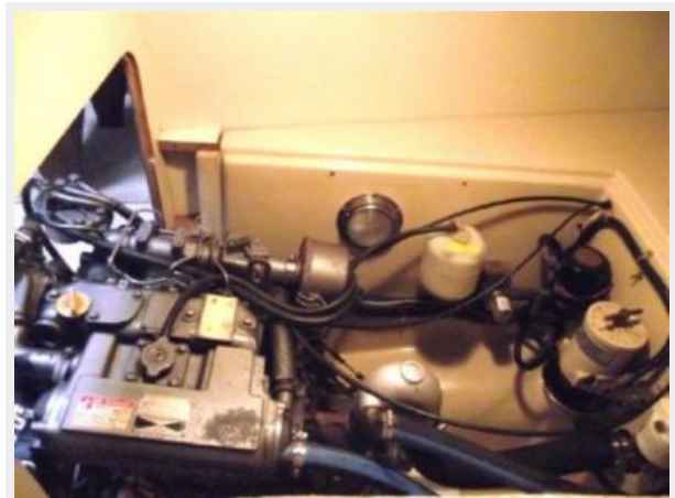
Clean engine room
