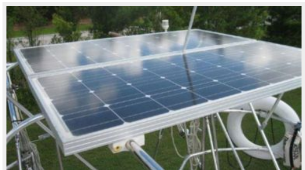
2X100 watt solar panels
