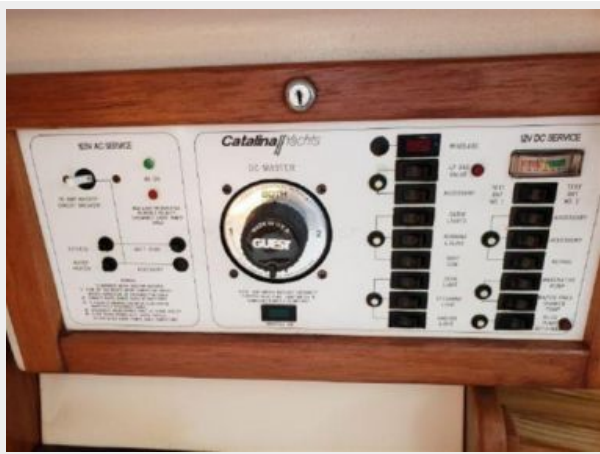
Electrical Panel at NavStation
