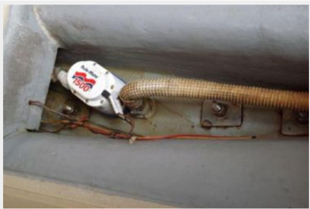
New Bilge Pump
