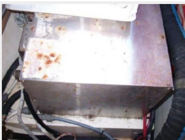
Seaward 6 Gal. Hot Water Heater
