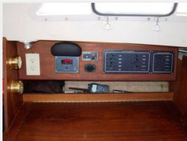
Electrical Panels & Nav Table
