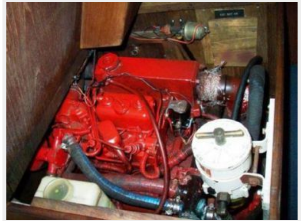
Westerbeke Diesel_Excellent Access
