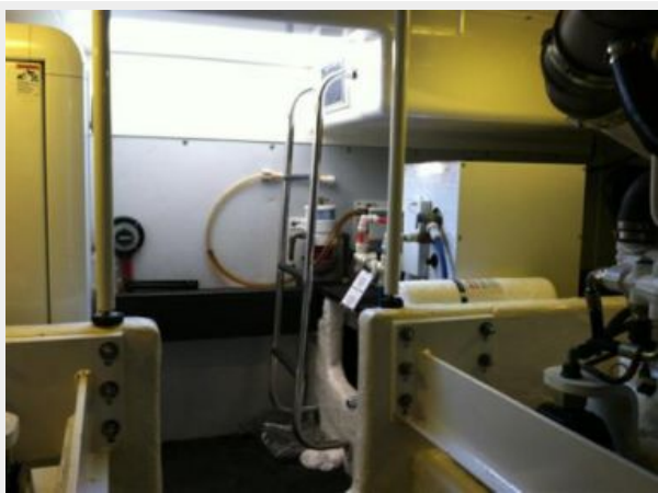
Charisma - Engine room aft
