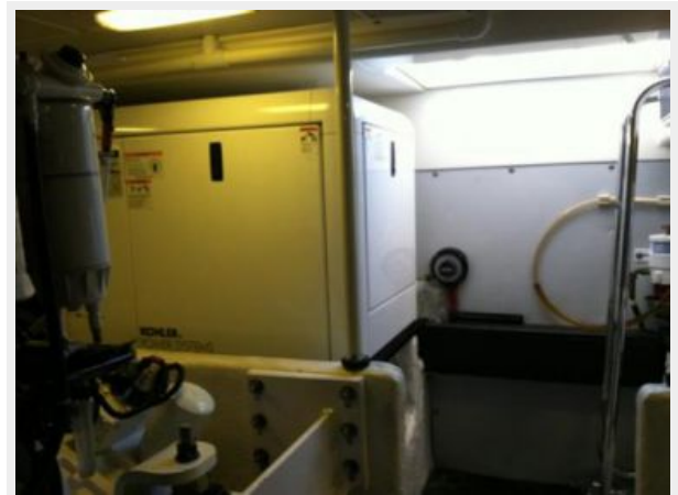
Charisma - 10 kw Generator
