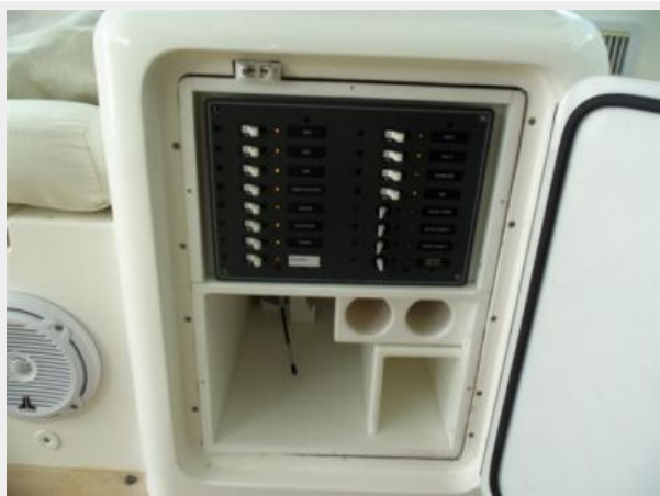
Helm Breaker Panel
