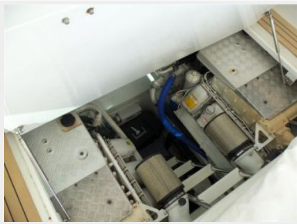
Helm Deck Engine Room Entrance
