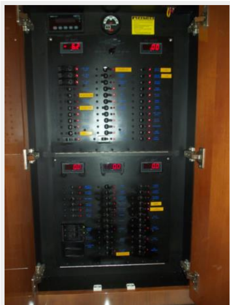
Galley Electrical Panel
