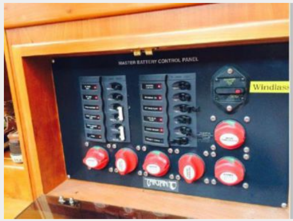
Battery Selectors Panel
