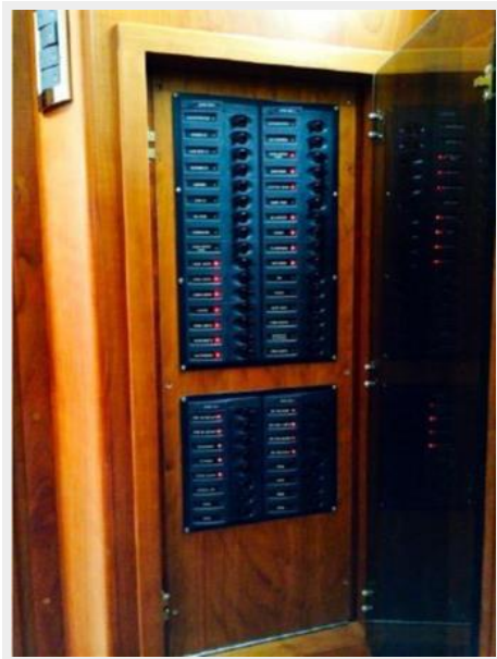
Breaker Panel Aft
