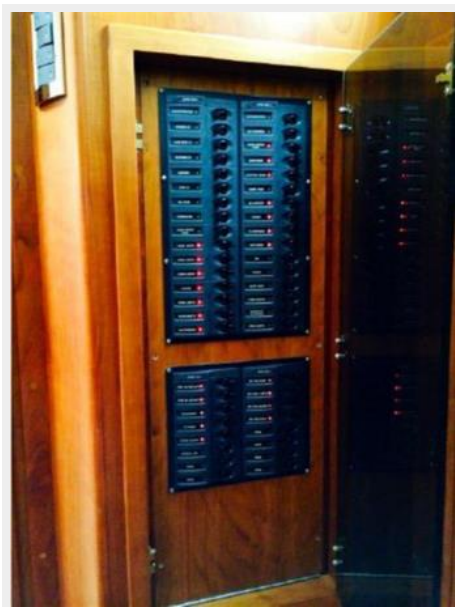
Breaker Panel Aft
