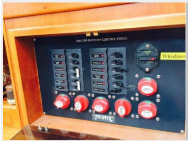
Battery Selectors Panel
