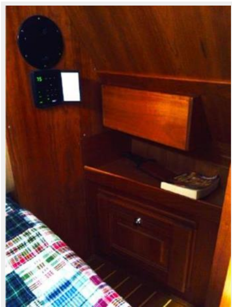
Aft AC Control
