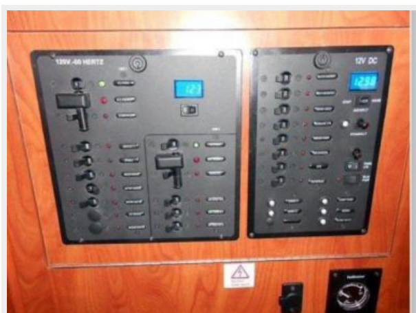
Electrical panel is tidy and hinged for easy service
