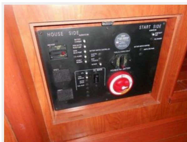
More electrical controls behind the panel under the seat
