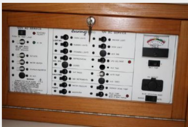
Electric breaker panel
