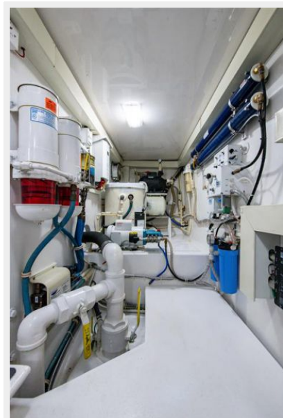
Paved For_Engine Room12
