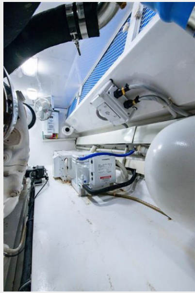
Paved For_Engine Room13
