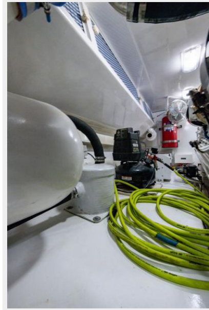
Paved For_Engine Room14
